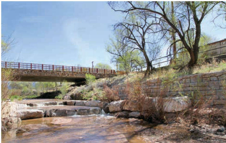
The retaining wall along the side of this stream is designed to reduce erosion due to water in the river channel.
